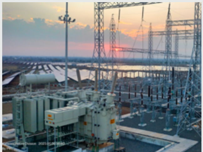
220 kV Switchyard, Khandwa
