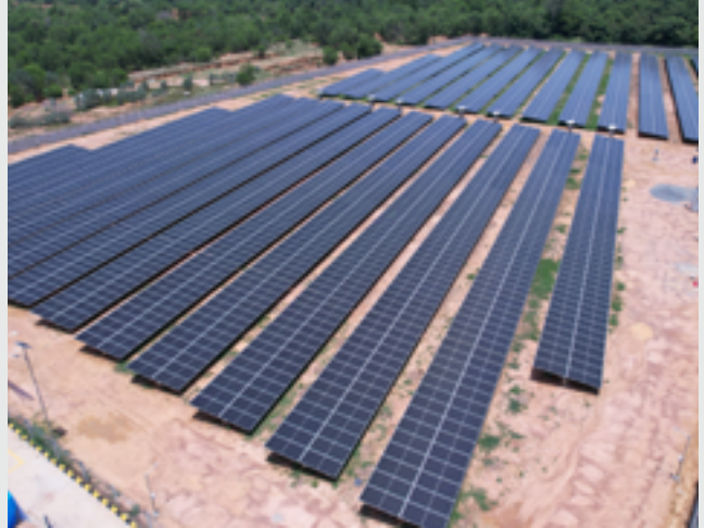
Daiki 2 MW Solar Plant, Sricity, Andhra Pradesh
