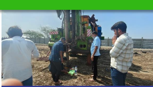
3.4 MWp Ground Mounted project (PM Kusum Yojna) at Chadchan, Karnataka
