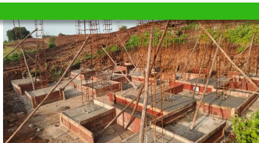
70 MWp Ground Mounted project at Jalna, Maharashtra
