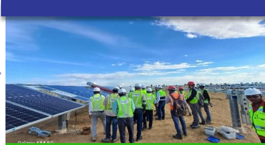
412.5 MWp Ground Mounted project at Bikaner, Rajasthan
