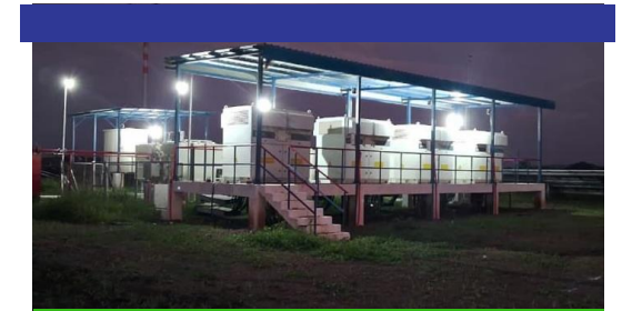
100 MWp Ground Mounted project at Jamnagar, Gujarat
