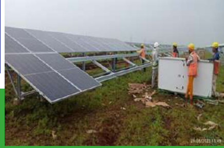
210 MWp Ground Mounted project at Khandwa
