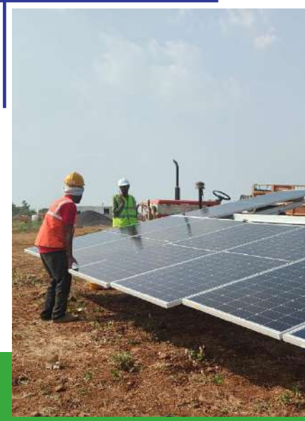
70MWp Ground Mounted project at Jalna
