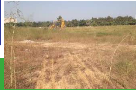
78MWp Ground Mounted Project at Tamnar, Chhattisgarh
