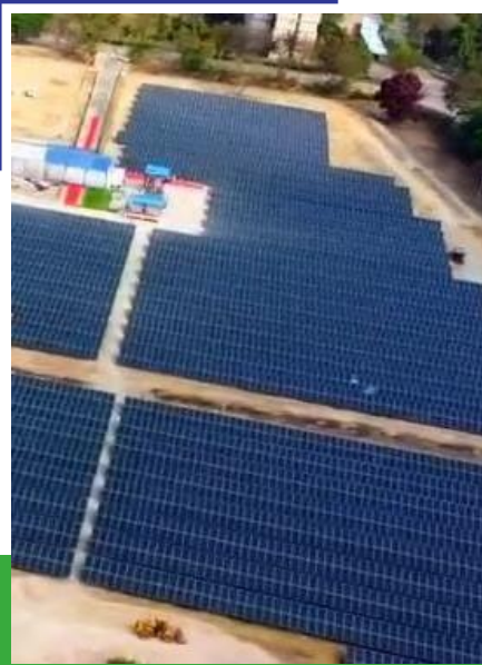
6.5MWp Ground Mounted Project at Raigarh, Chhattisgarh
