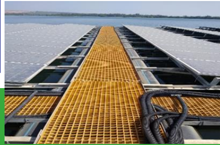
6.62MWp Rooftop project at Shri Godiji Plant, Chikhli
