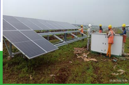
210 MWp Ground Mounted project at Khandwa
