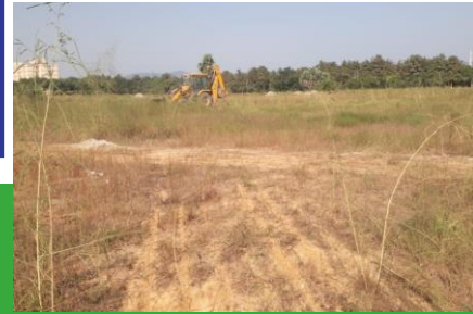
78MWp groundmount Project at Tamnar, Chattisgarh
