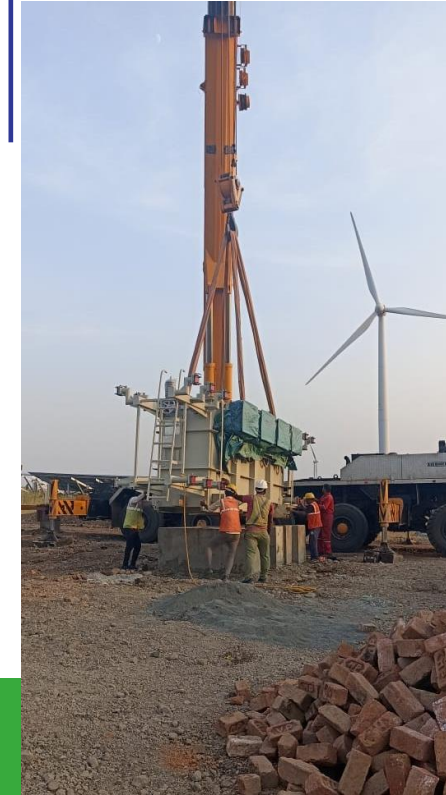
150MWp groundmount project at Ratlam, Madhya Pradesh
