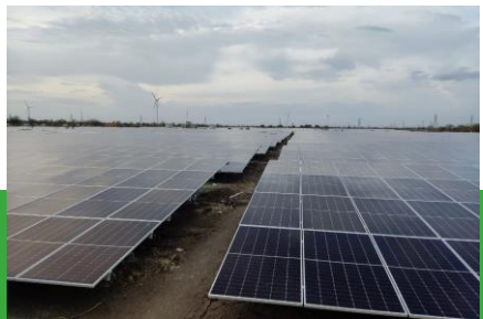
154 MWp ground mount project at Tamil Nadu
