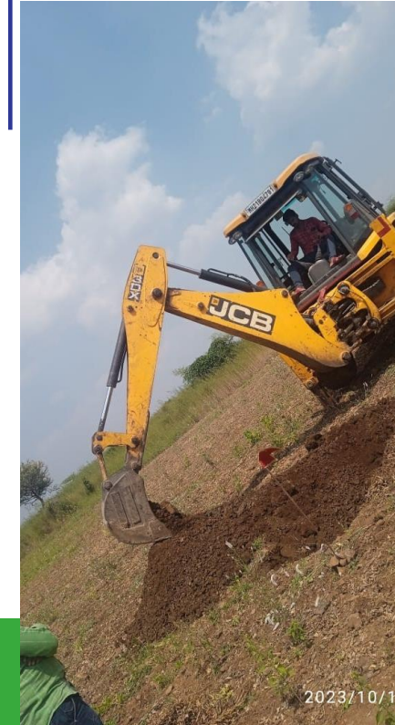
70MWp groundmount project at Jalna
