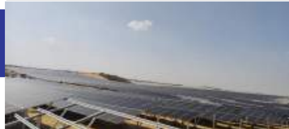
435 MWp Ground Mounted project at Bikaner, Rajasthan
