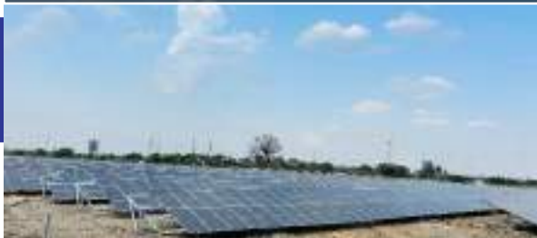
105 MWp Ground Mounted project at Jamnagar, Gujarat
