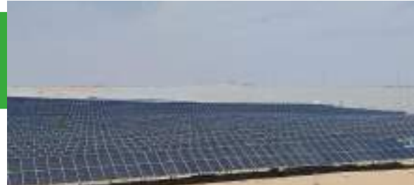
450 MWp Ground Mounted project at Bikaner, Rajasthan
