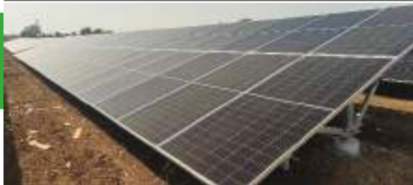
131 MWp Ground Mounted project at Nashik, Maharashtra
