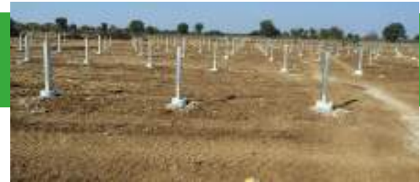
29.4 MWp Ground Mounted project at Yavatmal, Maharashtra
